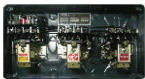
Interior View of MK1 SASD
