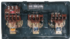
Interior View of MK2 SASD
