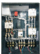
Interior View of MU-G30W FASD
